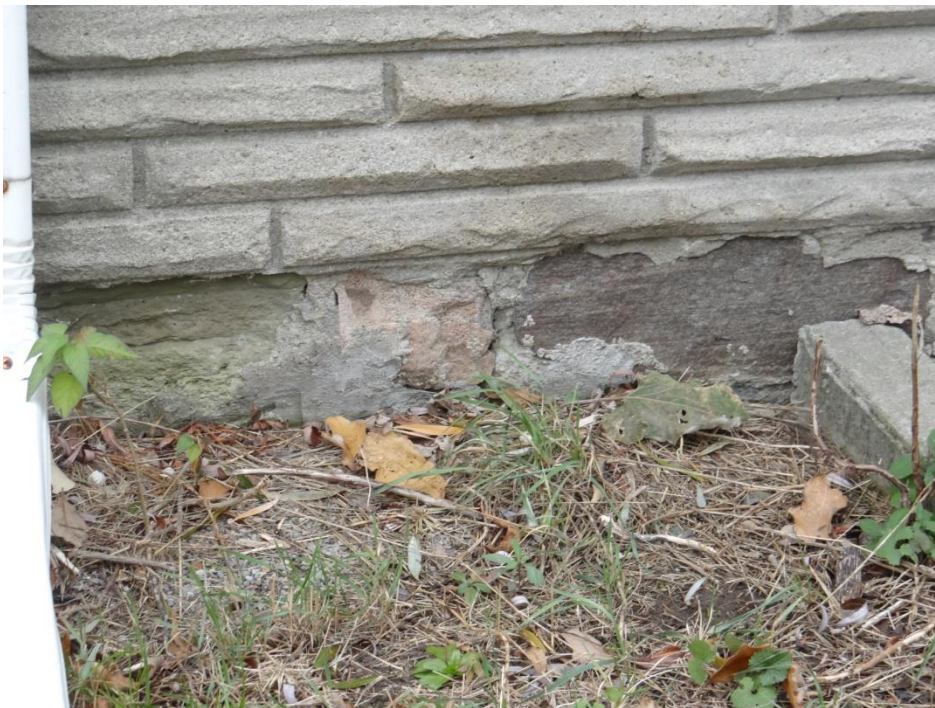
Plate 4: Detail of the foundation where the cladding has spalled, exposing the field stone beneath (northeast corner)
