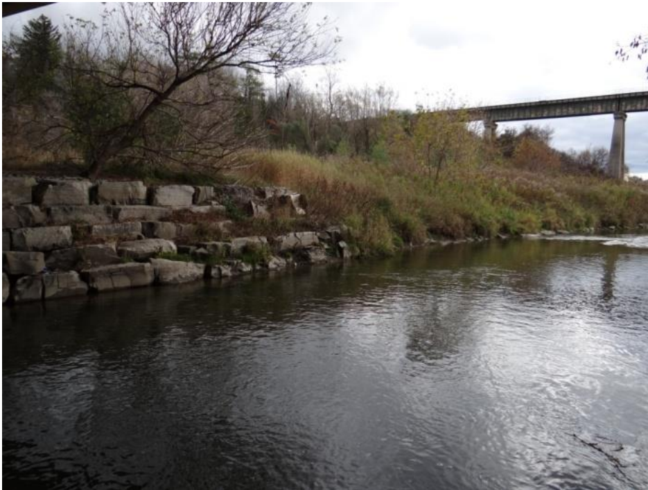
Plate 9: Limit of stepped stone bank stabilization to south of bridge, looking southeast.
